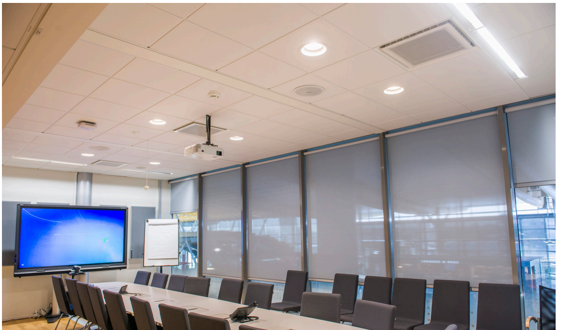
OSLO AIRPORT GARDERMOEN, NORWAY DID-614
