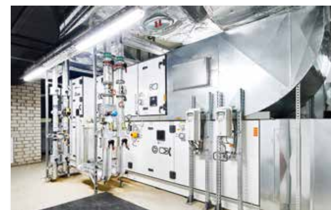
An air handling unit with an intelligent control system provides air based on demand.
